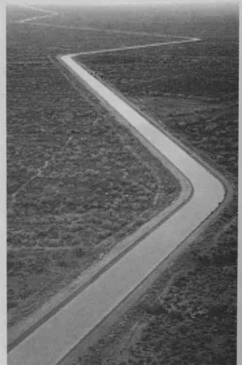
Central Arizona Project Canal, west of Phoenix, Arizona. (Photograph by Darryl Webb, Mesa Tribune, published with permission.)
