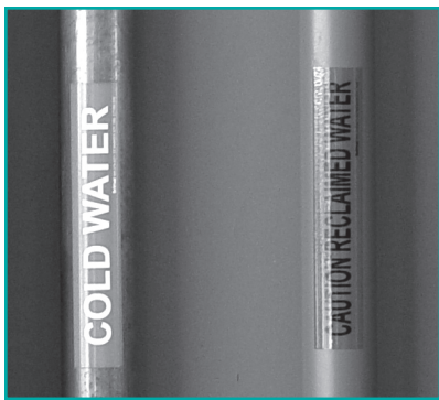
Purple pipes: a dual piping system is used in the City of Maricopa to keep reclaimed water and potable water separate. Source: Channah Rock.
