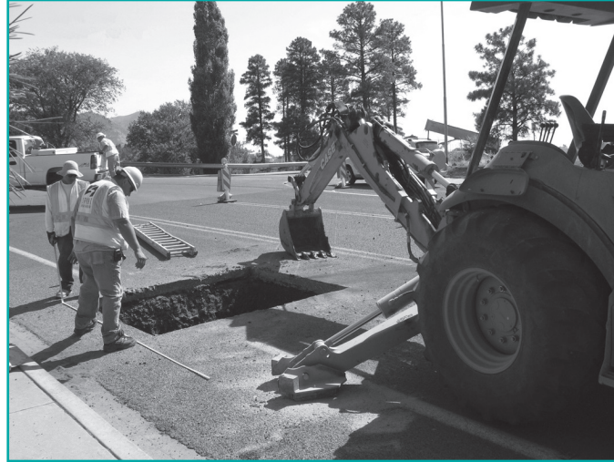
Trenching to bring reclaimed water service to new commercial development in Flagstaff. Source: Aspen Sawmill Project.
