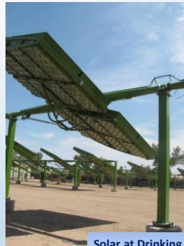
Solar at Drinking Water Facility City of Somerton
