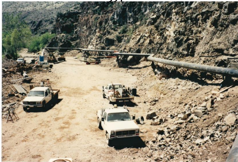
24" steel welded aerial line.
