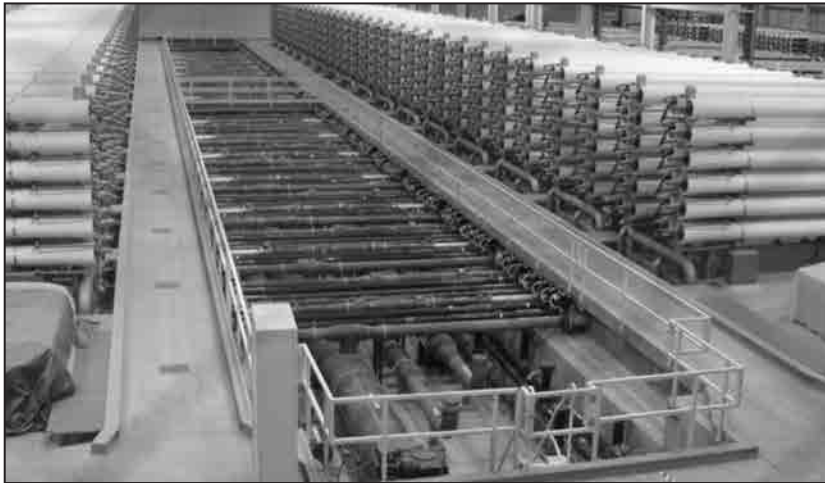
Banks of reverse osmosis membranes at the Yuma Desalting Plant. Source: Placido Dos Santos
