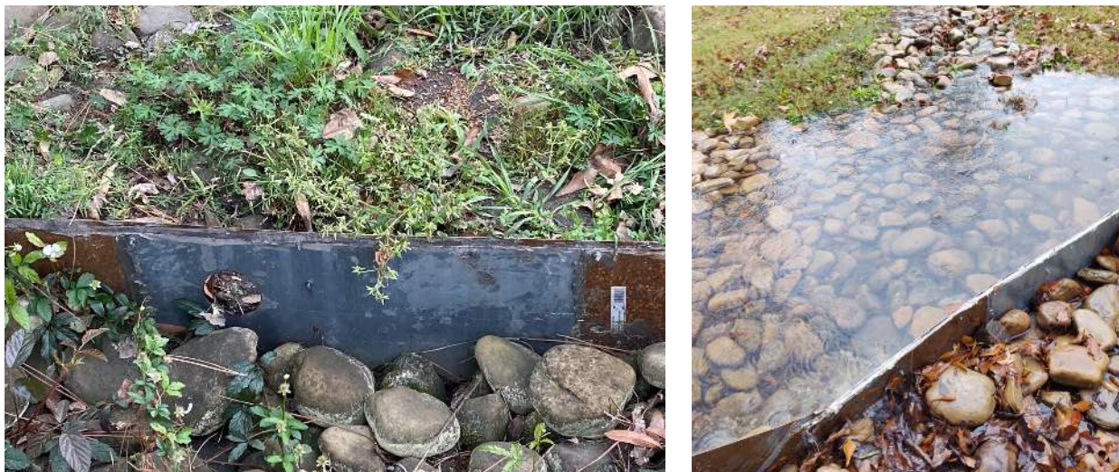
Figure 2. Hydraulic structure at the entrance to the bioretention basin with an orifice for low-flow measurement and a weir for high-flow measurement.
