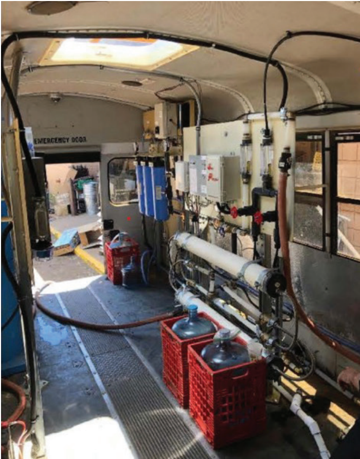
Decentralized nanofiltration display in the Apex Applied Technology "Water Bus." Image: Apex Applied Technology, Inc.
