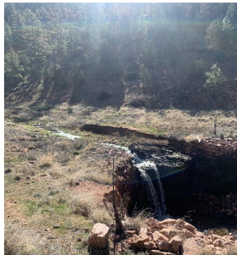
Figure 3: In 2023 after the repair failed.
