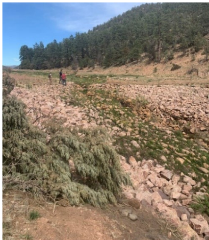
Figure 2: First headcut repair in 2011. (Shown here 10 yrs after initial repair in 2022)
