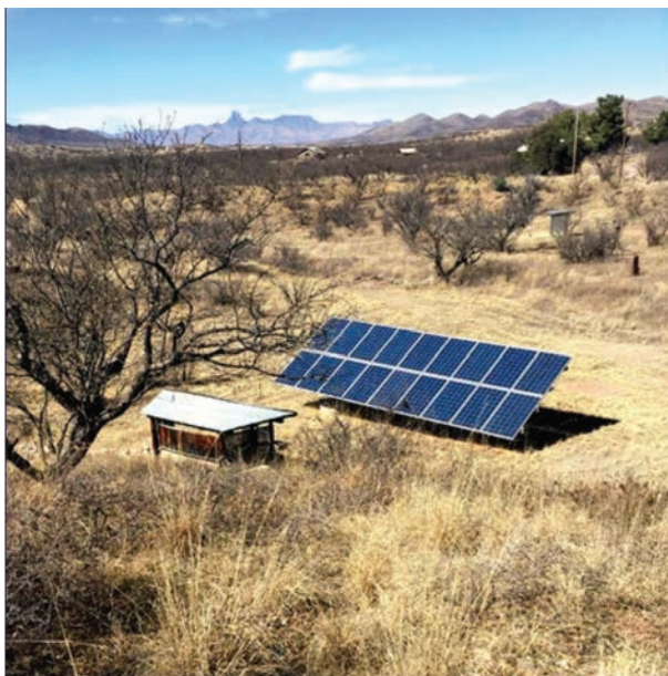
Figure 8.11 Domestic well powered by Solar cells. Source: Artiola, Uhlman, Hix, 2017. Arizona Well Owner's Guide to Water Supply 2 nd Edition .
