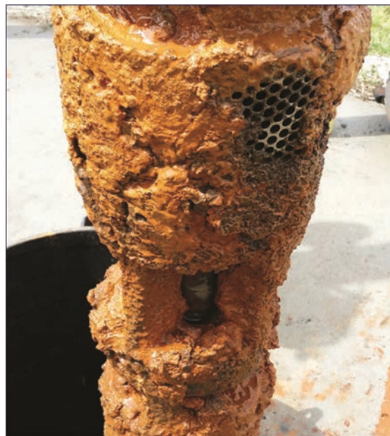
Figure 4.1 Buildup of biological slime and mineral crust on a submersible pump inlet. Source: Gary Hix
