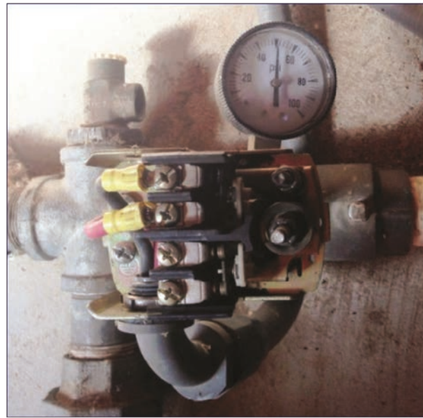
Figure 3.8 Captive air bladder tank pressure switch. Source: Artiola, Uhlman, Hix, 2017. Arizona Well Owner's Guide to Water Supply 2 nd Edition
