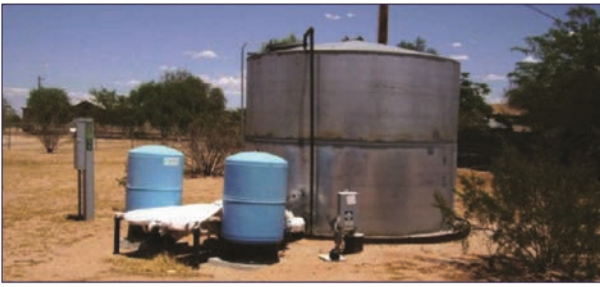
Figure 3.9 A shared well system with above ground storage and two pressure tanks, delivering water to two households. Source: Artiola, Uhlman, Hix, 2017. Arizona Well Owner's Guide to Water Supply 2 nd Edition
