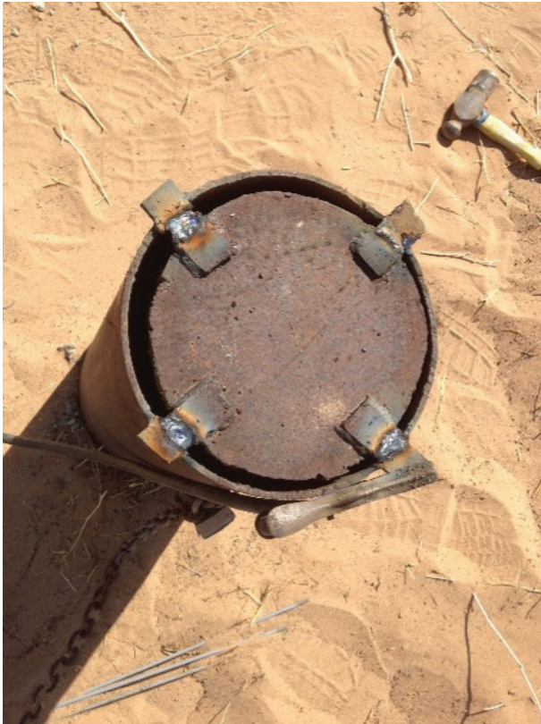
Figure 9.3 Photo of an improperly capped unused well that should be abandoned. Improperly abandoned wells can be a source of groundwater pollution and maybe a safety concern. Source: Gary Hix
