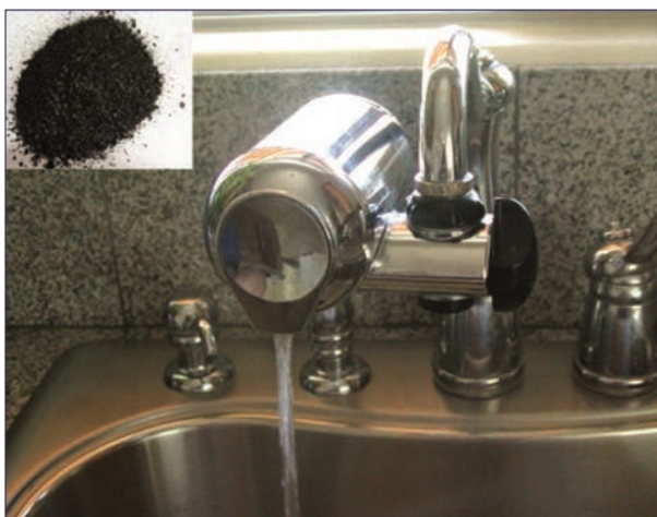
Figure 8.5 An activated carbon point-of-use treatment installed on a faucet; the carbon media is shown in the photo insert. Source: Artiola, Uhlman, Hix, 2017. Arizona Well Owner's Guide to Water Supply 2 nd Edition .
