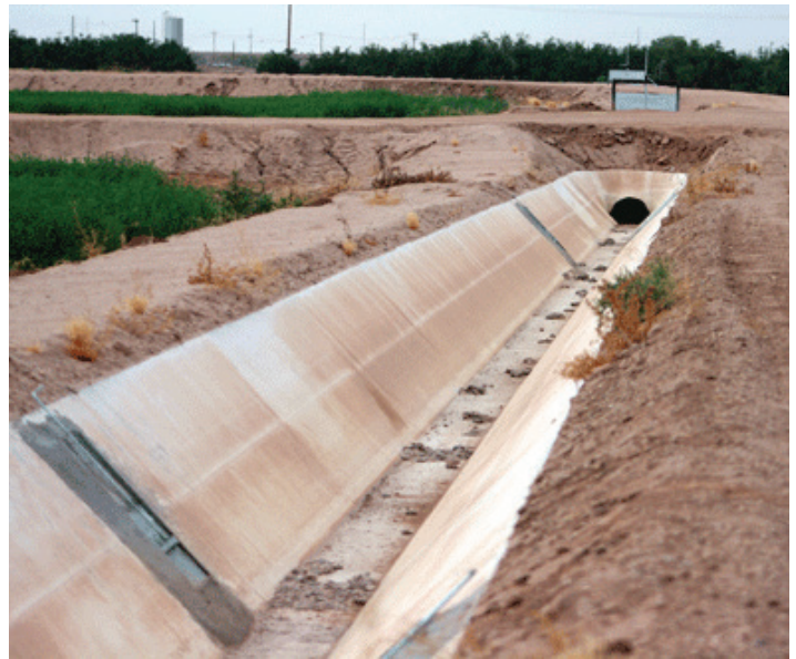
Lined irrigation ditches installed at Morning Star Farms in Florence, Arizona, to improve irrigation efficiency. Source: National Resources Conservation Service
